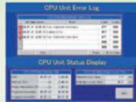
PLC CPU Unit monitoring screen
